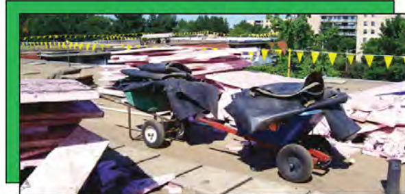
A "before" photo in the roofing process, as an old rubber roof is torn off before a new one is put in its place.
